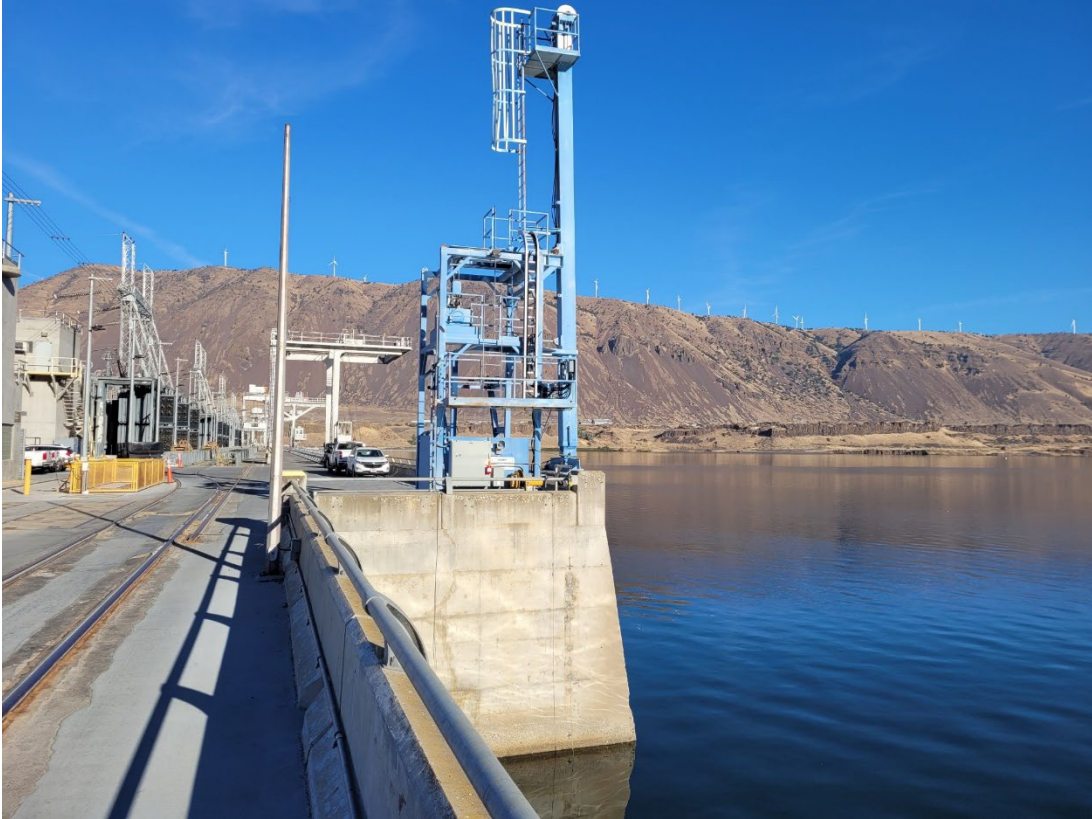
Fig 1. The John Day penstock trash rack crane.
